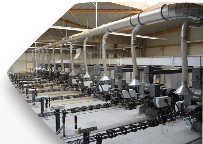
Installation of Holzindustrie Torgau, Germany
